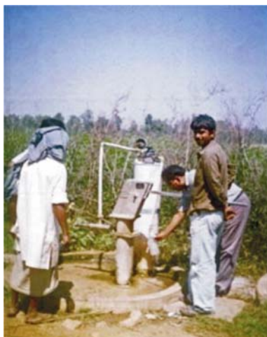
Figure 6. Handpump attached defluoridation plant lying dysfunctional due to absence of O&M in Palamau district of Jharkhand state.
